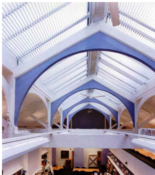
Internal T50 fitted in library
